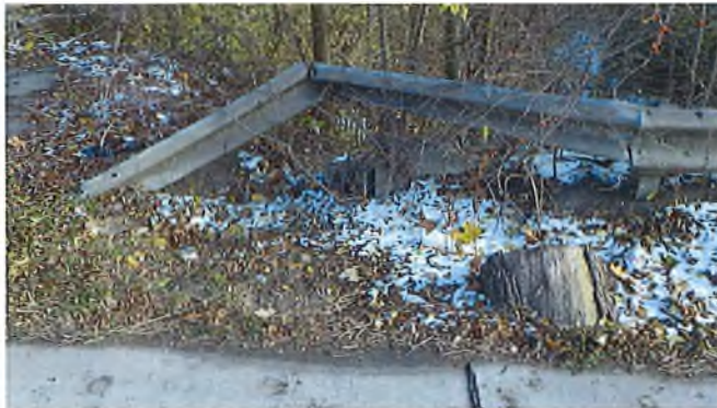
Document Name: RIMG2897.JPG Category: Railing Span Number: Comments: NE guardrail end damaged and dates back to 2016
