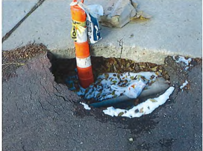
Document Name: RIMG2877.JPG Category: Other Span Number: Comments: 2'x3'x2'deep sinkhole just north of culvert, along driveway to the east.
