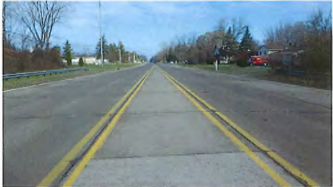
Document Name: RIMG2977.JPG Category: Approach Span Number: Comments: north approach looking north
