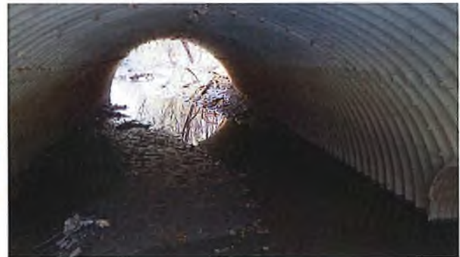
Document Name: RIMG2883.JPG Category: Culvert Span Number: Comments: North Barrel of Culvert
