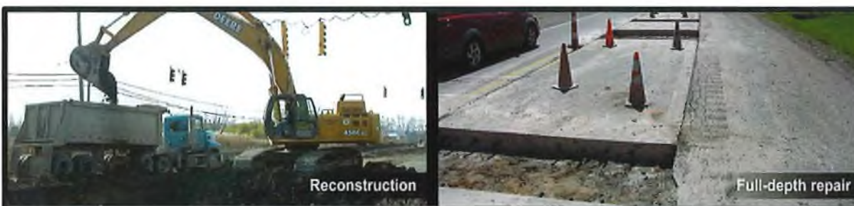
Figure 0-2. Examples of Reconstruction Treatments—(left) Reconstructing a Road and (right) Road Prepared for Full-Depth Repair
