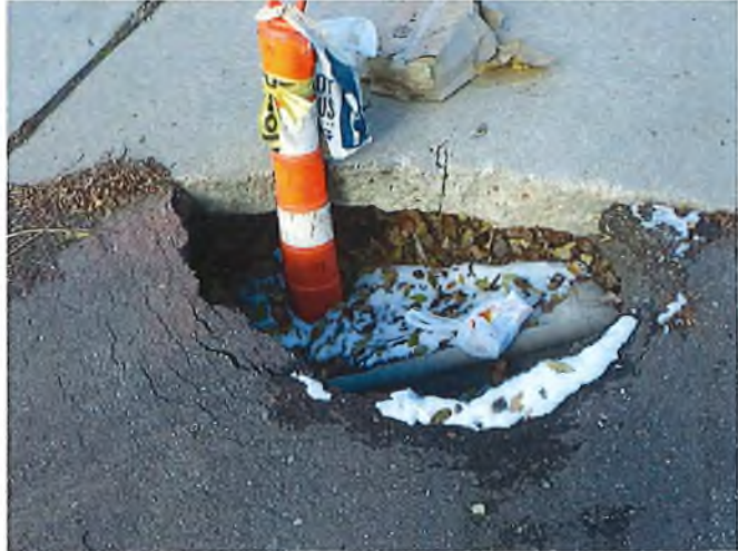
Document Name: RIMG2877.JPG Category: Other Span Number: Comments: 2'x3'x2'deep sinkhole just north of culvert, along driveway to the east.
