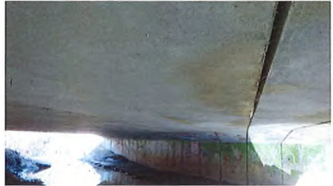
Document Name: RIMG3070.JPG Category: Culvert Span Number: Comments: 3E is displaced 1/4" down
