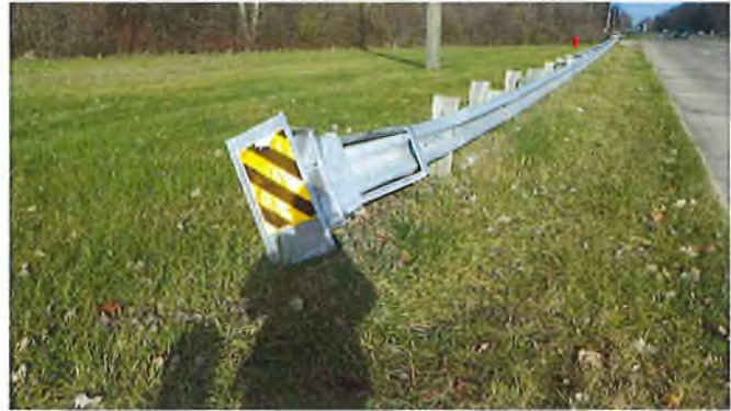
Document Name: RIMG3004.JPG Category: Railing Span Number: Comments: SW guardrail impact attenuator damage.
