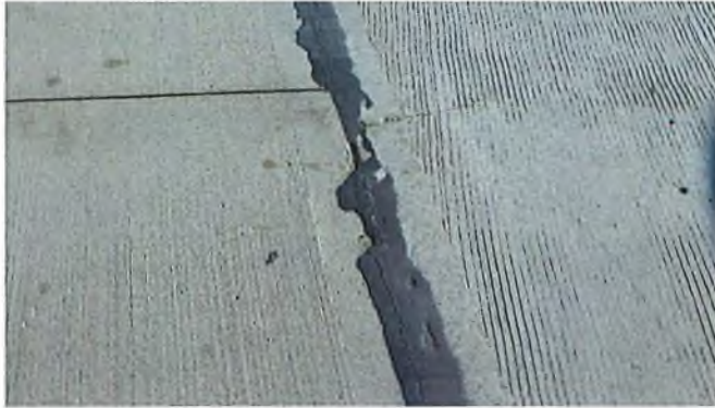
Document Name: RIMG3021.JPG Category: Joints Span Number: Comments: Missing sealant at mid-span in joint
