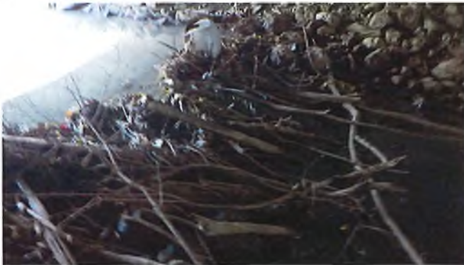
Document Name: RIMG2996.JPG Category: Channel Span Number: Comments: view of dam blocking channel
