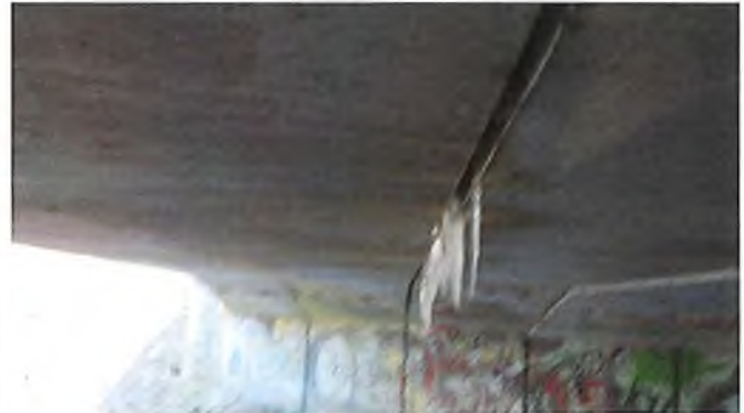
Document Name: RIMG3078.JPG Category: Culvert Span Number: Comments: Leaking between 2W and 3W 1" settlement between 3W and 4W
