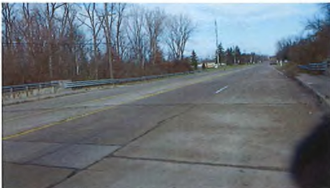
Document Name: RIMG2966.JPG Category: Approach Span Number: Comments: South approach looking north
