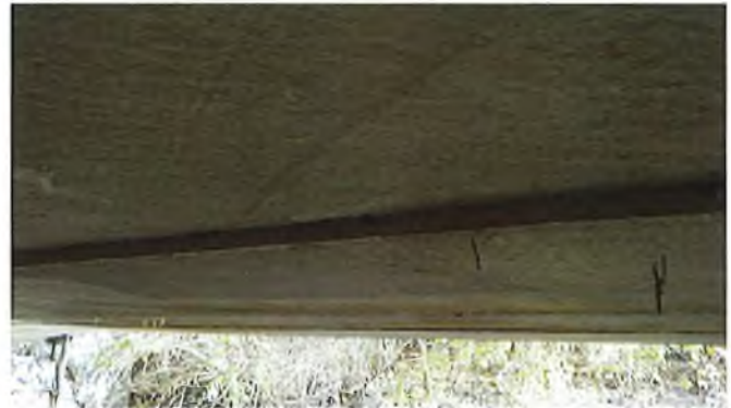
Document Name: RIMG3073.JPG Category: Culvert Span Number: Comments: 1" gap between beams 3E and 4E
