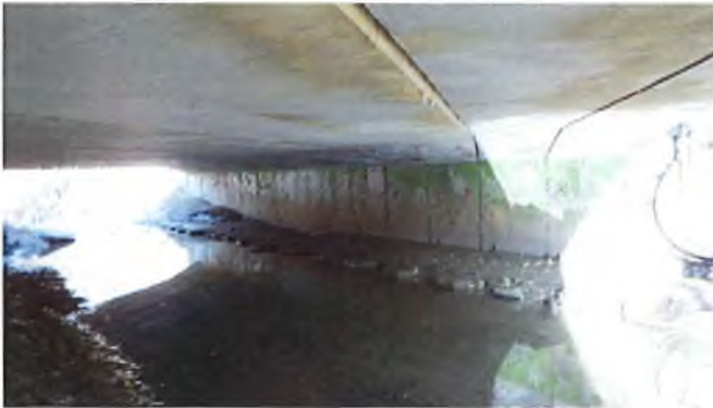
Document Name: RIMG3071.JPG Category: Culvert Span Number: Comments: 3E is displaced 1/4" down 1" gap between beams 3E and 4E
