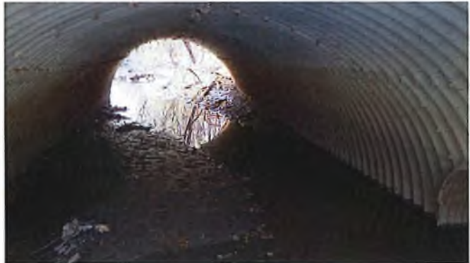
Document Name: RIMG2883.JPG Category: Culvert Span Number: Comments: North Barrel of Culvert
