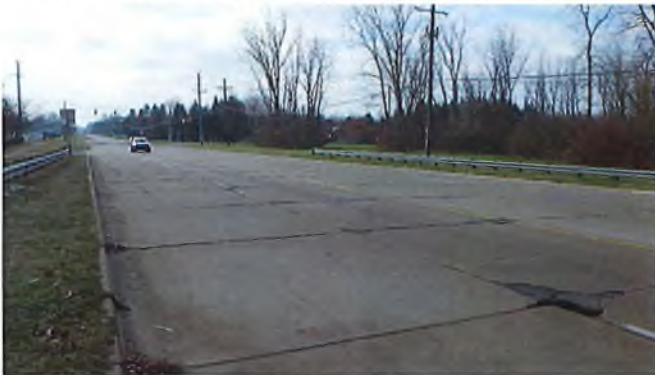
Document Name: RIMG2967.JPG Category: Deck Span Number: Comments: typical view of deck
