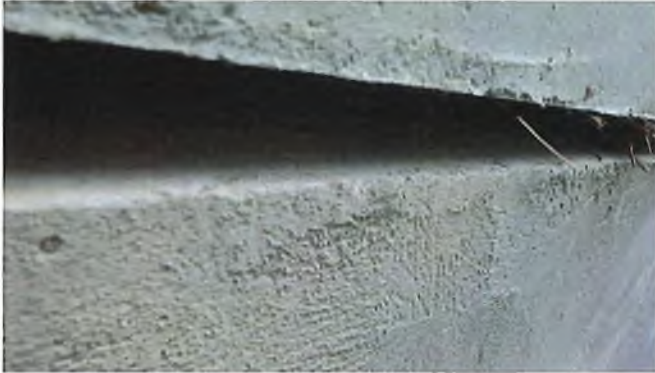
Document Name: RIMG3074.JPG Category: Culvert Span Number: Comments: 1" gap between beams 3E and 4E
