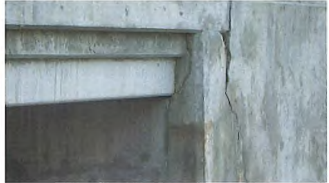
Document Name: RIMG3044.JPG Category: Substructure Span Number: Comments: SW quad has spall/crack
