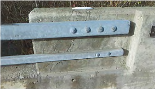
Document Name: RIMG2981.JPG Category: Railing Span Number: Comments: 4 ft long diagonal through crack at Northwest end wall at metal railing anchorage point with concrete end wall
