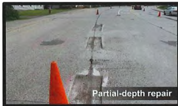
Figure 0-5. An Examples of Capital Preventive Maintenance Treatment is Concrete Road Prepared for Partial-Depth Repair.
