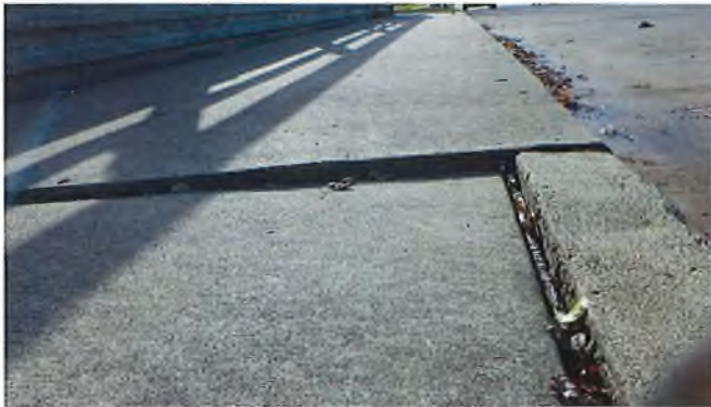
Document Name: RIMG3046.JPG Category: Approach Span Number: Comments: typical view of trip hazard at sidewalk approaches
