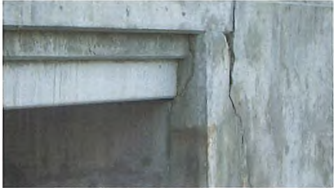
Document Name: RIMG3044.JPG Category: Substructure Span Number: Comments: SW quad has spall/crack
