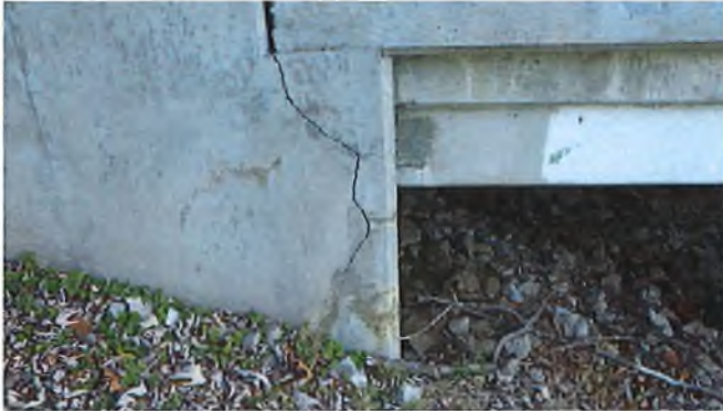
Document Name: RIMG3042.JPG Category: Substructure Span Number: Comments: Vertical cracks at interface of wingwall and abutment
