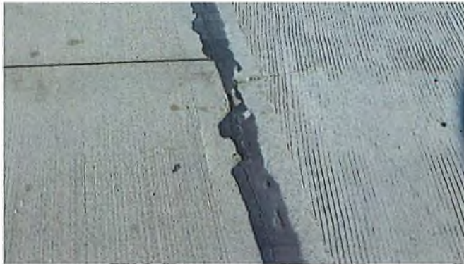
Document Name: RIMG3021.JPG Category: Joints Span Number: Comments: Missing sealant at mid-span in joint
