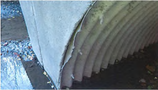
Document Name: RIMG2885.JPG Category: Culvert Span Number: Comments: Damage to North barrel at headwall
