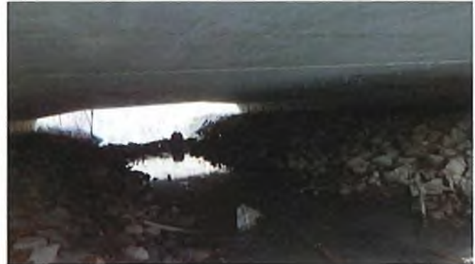
Document Name: RIMG2995.JPG Category: Channel Span Number: Comments: View of dam under culvert
