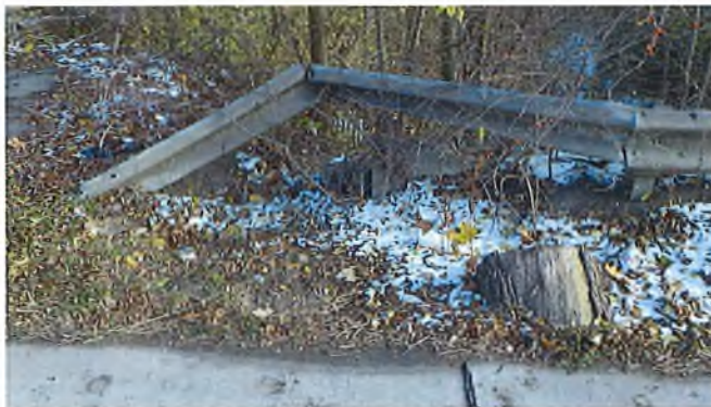
Document Name: RIMG2897.JPG Category: Railing Span Number: Comments: NE guardrail end damaged and dates back to 2016
